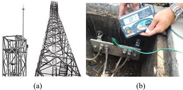
Gambar 4.12 Grounding tower (a) bak kontrol (b)
