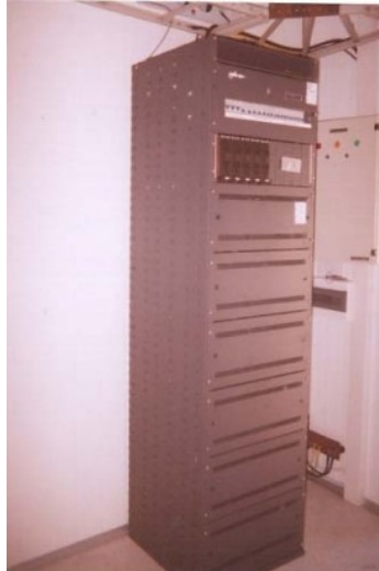
Gambar 3.23 Rectifier Power One PPS16.48[12]
