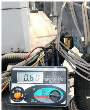
Gambar 4.14 Hasil pengukuran grounding
