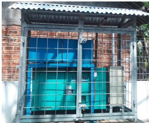
Gambar 4.32 Genset permanen (statis)
